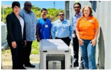
Little Cayman standby generator
